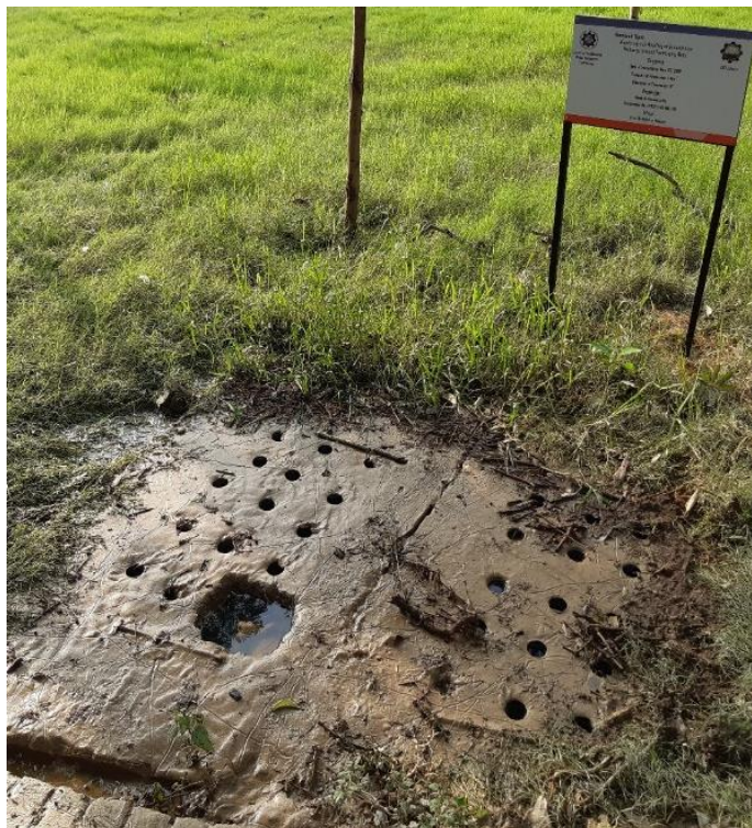
Figure 4.9 Ponding situation on July 17, 2019 due to Rainfall occurred on July 16, 2019
