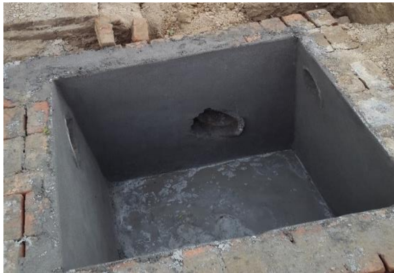
Figure 2.12 Sump for Desiltation
