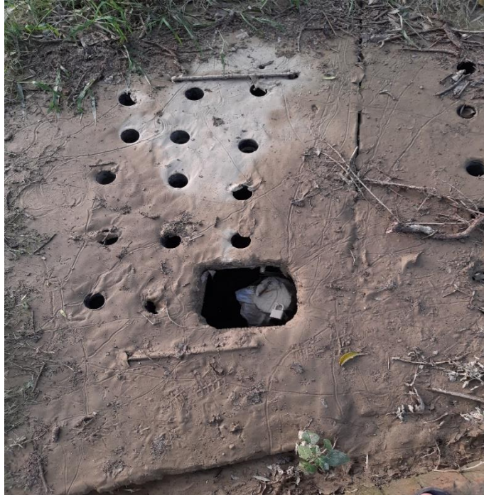
Figure 4.10 Ponding situation on July 18, 2019 due to Rainfall occurred on July 16, 2019
