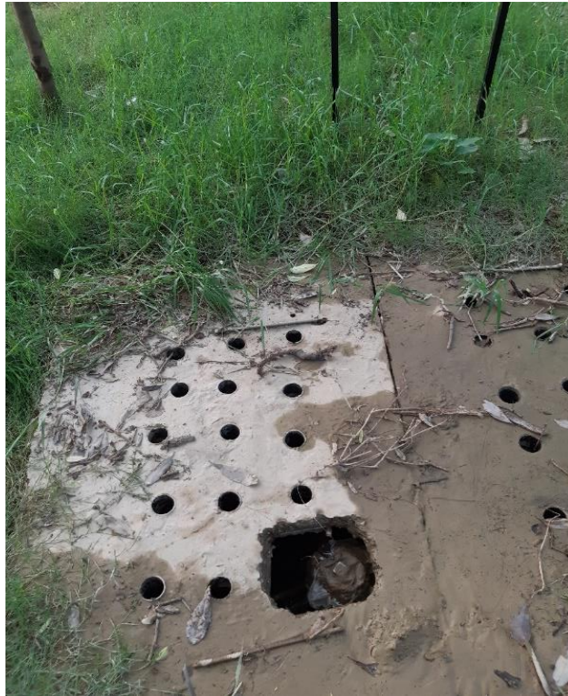
Figure 4.12 Ponding situation on July 26, 2019 due to Rainfall occurred on July 25, 2019
