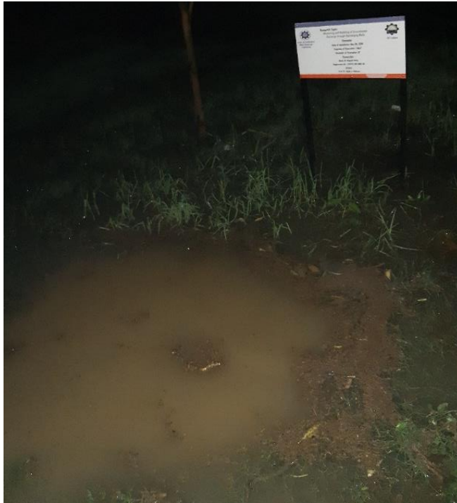
Figure 4.8 Ponding on Sump connected to RW2 after Rainfall on July 16, 2019
