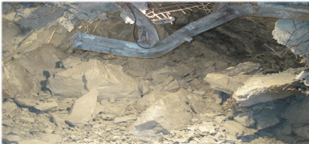
Figure 1.1: Rock burst damage in a hydropower tunnel (After Yu, et al., 2015)
